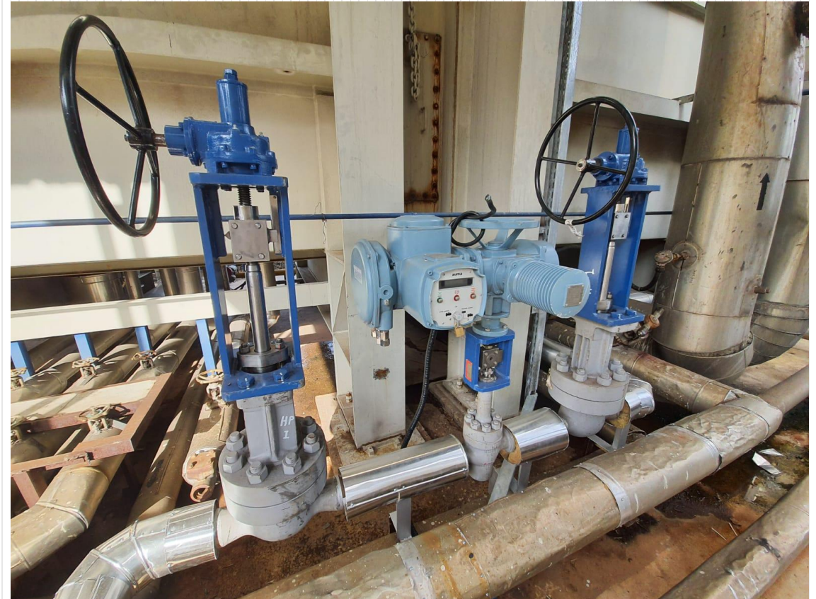
HP - LP Drain Valve PLTGU Gunung Megang - South Sumatra
